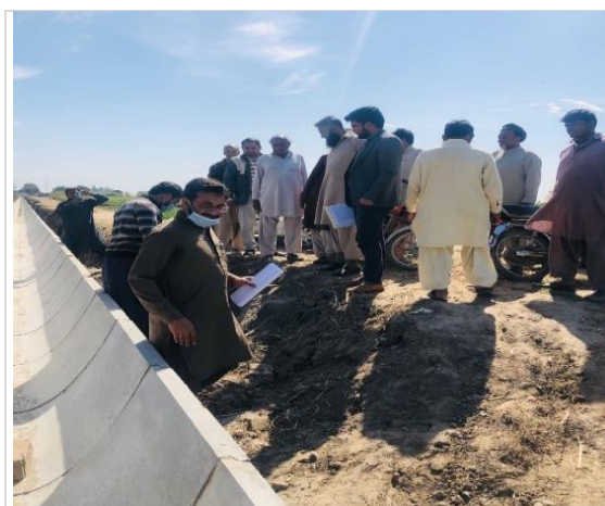
Figure 4.15: Site Visit at 12648 R Under Construction Watercourse along with Supervisor and Beneficiaries
